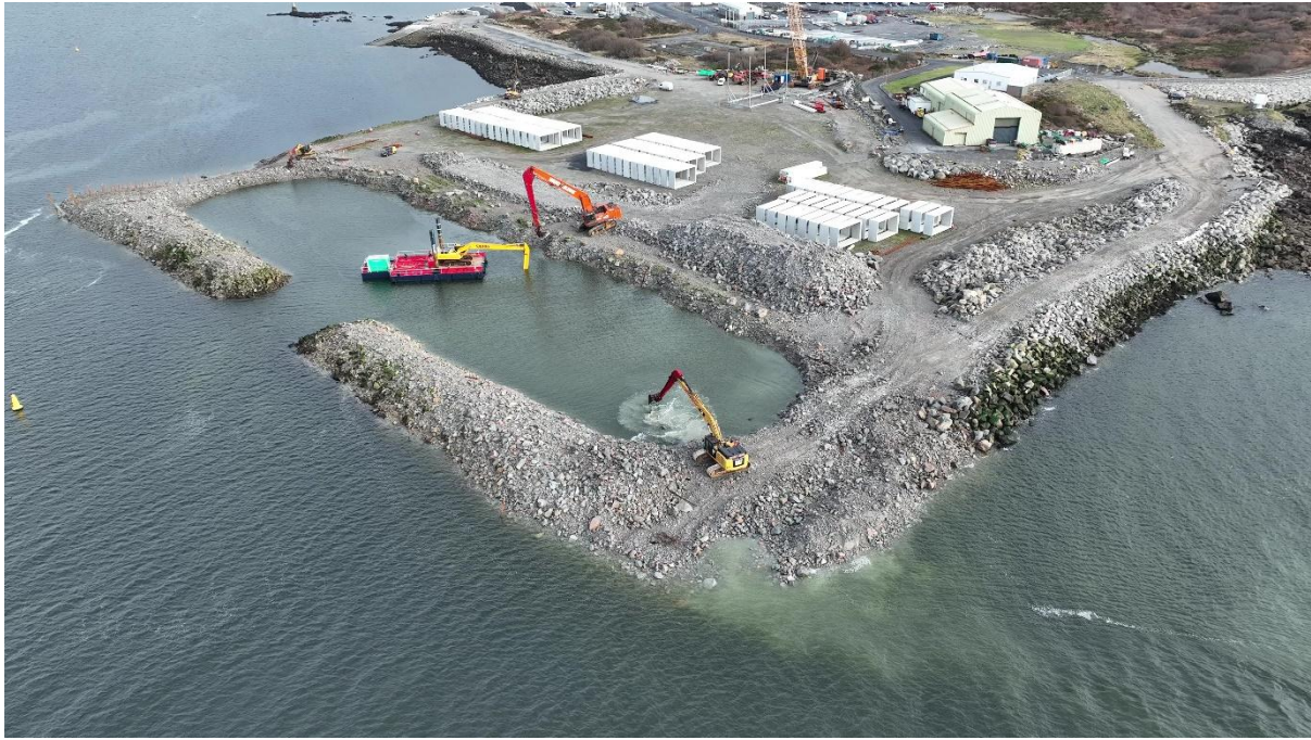
Figure 15-1: Excavators working behind a semi-enclosed stone bund in Ros an Mhíl, Co. Galway
